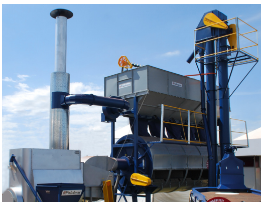
Silos superiores de pre-secado ( https://bit.ly/3tk6D4Z )
