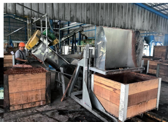
Illustrative photos of the equipment installed
